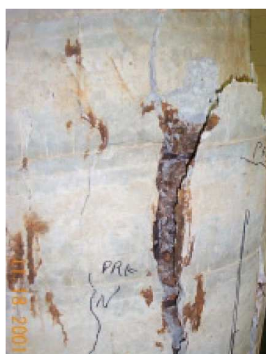
Fig. 2.41 Fracture of cover concrete induced by buckling of vertical reinforcement in compression (Aquino 2002)
