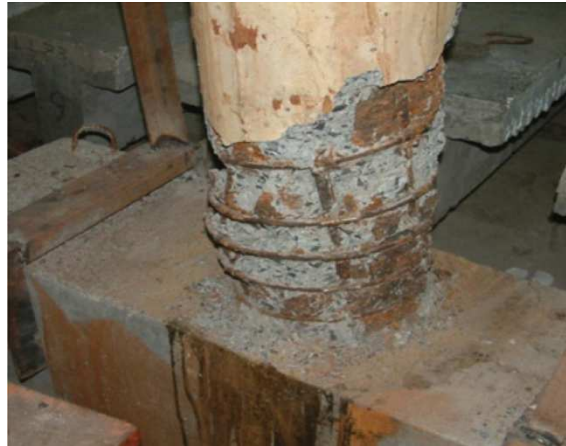
Fig. 2.46 buckling of vertical reinforcement in specimen C14-32 with 14.7% mass loss and axial force ratio of 0.32 (Ma et al. 2012)
