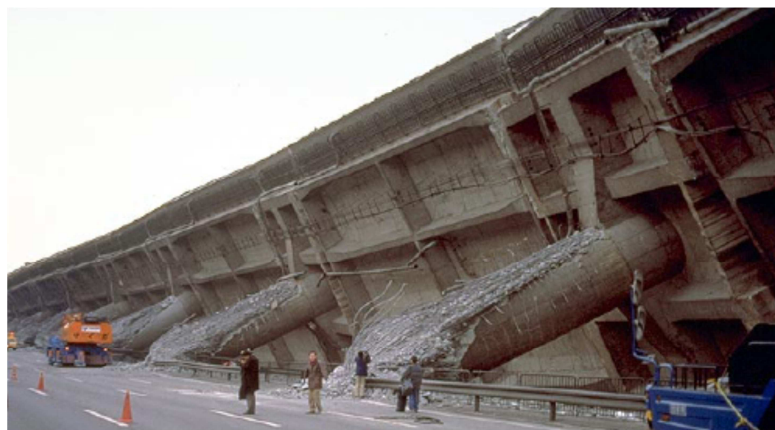
Fig. 1.4 Collapse of a RC bridge in Kobe earthquake due to lack of confinement and buckling of vertical reinforcement (Arscott 1995)
