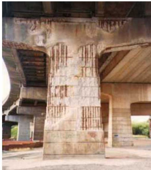
Fig. 1.3 Corrosion damaged RC bridge pier (Lambert and Atkins 2007)
